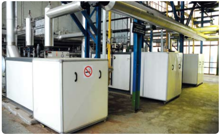
Modern gas-fired boilers at the city campus.
